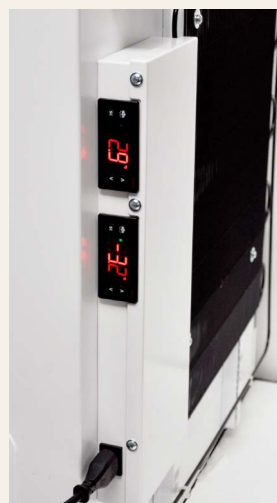
Controller junction box
