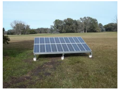
PV for pumping water
