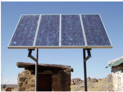
PV on farm in Córdoba
