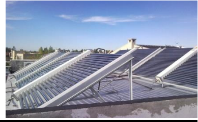
Heating water facilities
