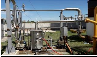
Supply equipment for biogás facility in Coca Cola Córdoba
