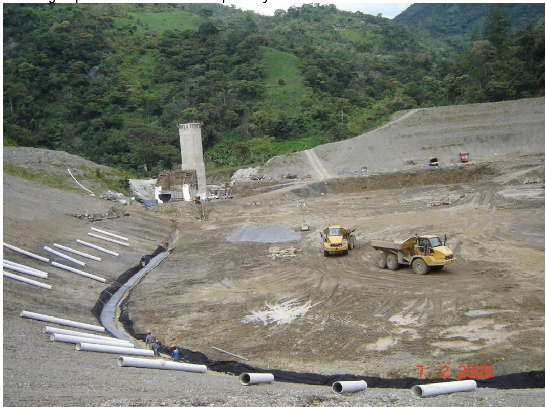
Hydroelectric Power Plants, MEP installations. Solel Boneh Int. Guatemala
